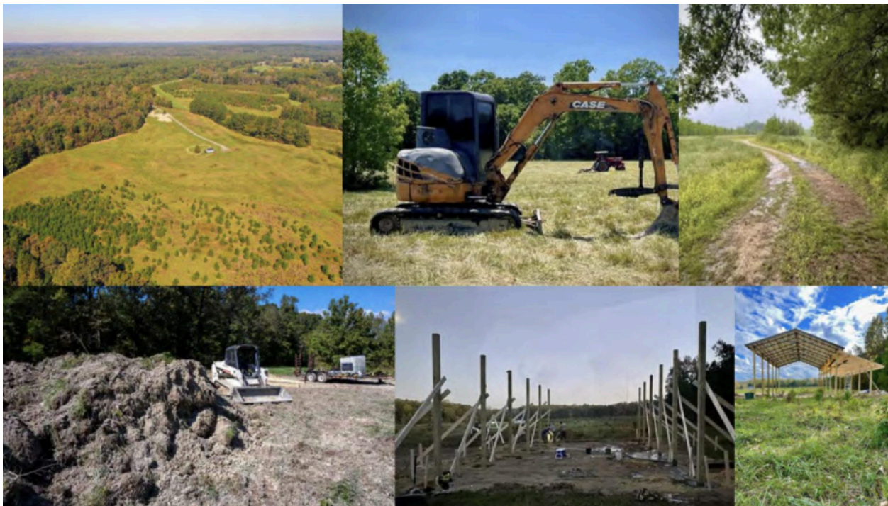
Construction of the sanctuary buildings is underway. Photo courtesy of Beautiful Together.
